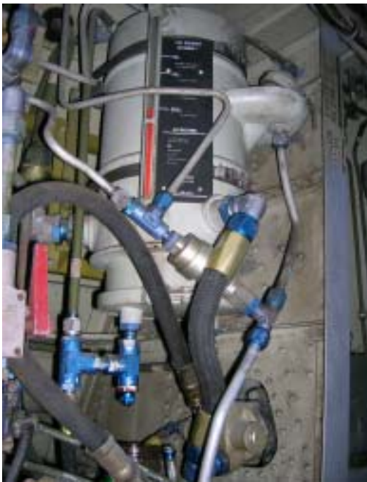
Hydraulic system reservoir.
